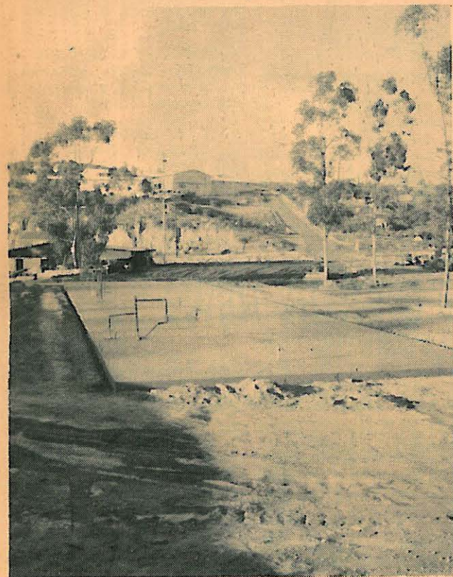
The cement slab poured Monday for the new apartment buildings on Arnold Way. In background is the filled area where Jerry Funk is planning to erect his new building. (Town and Country photo)
